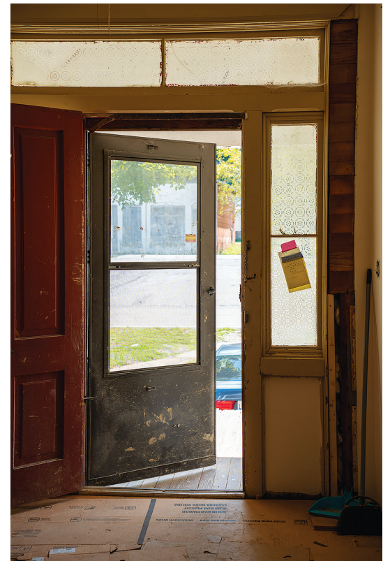
During Hurricane Helene, Theo Crouse-Mann's home in Del Rio, Tennessee, suffered extensive flood damage from the French Broad River. Photo by Abby Hassler
