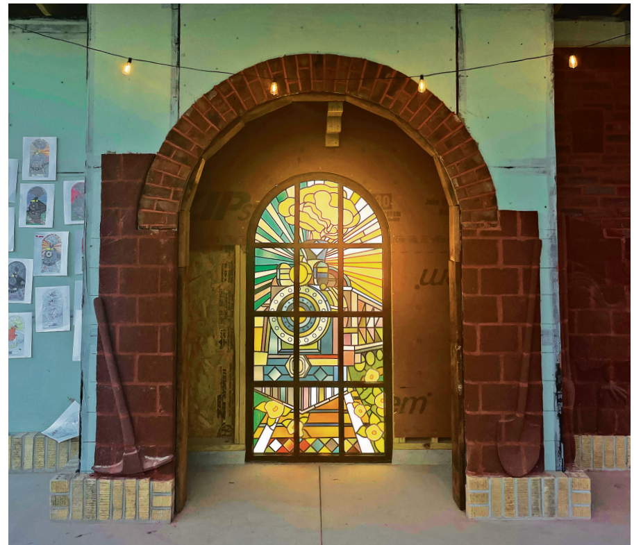
Stained-glass art, representing a nearby tunnel once used by coal trains, centers the new stage being built in Pound, Va. The stage will serve as a monument to the town's labor history as well as a local gathering place. Photo by Kara Dotten
