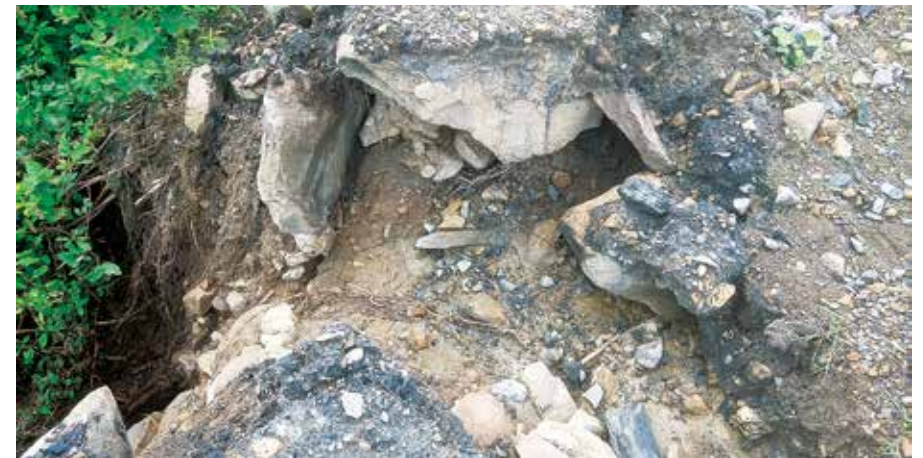
The ditches meant to contain runoff from the unreclaimed Aily Branch mine are clogged with sediment, which caused this berm to burst and send a torrent of mud and debris toward the Mitchells' home this summer. Below, a mine permit sign. Photos by Willie Dodson
