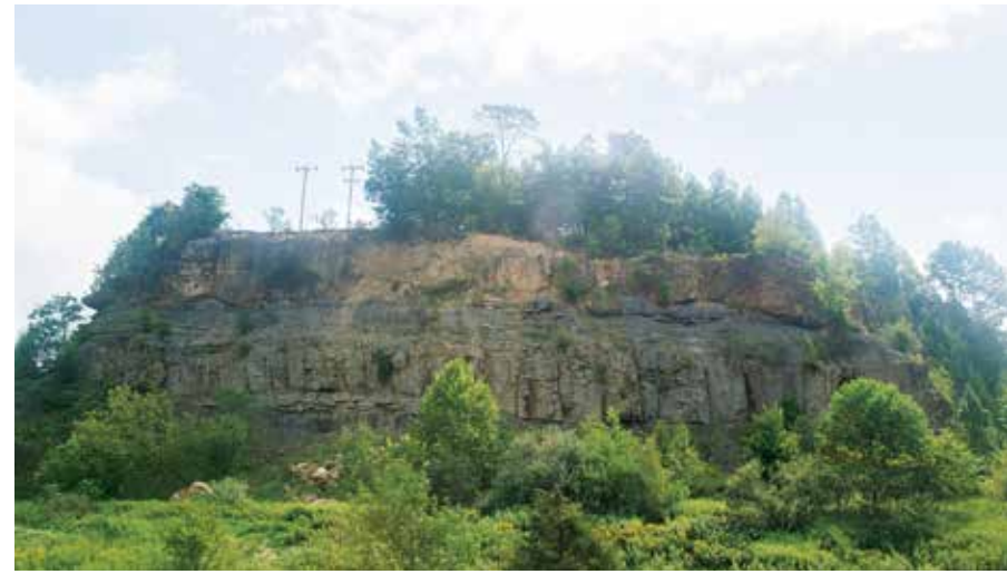
Officials plan to remove this dangerous highwall next to a four-lane highway in Norton, Va., as part of an AML Pilot project. Photo by Kevin Ridder
