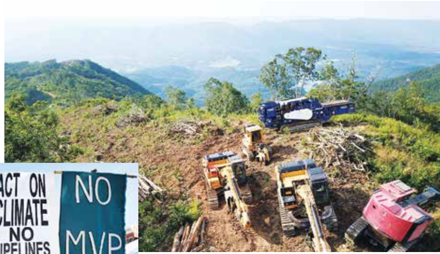
Above, MVP Construction near Virginia's Poor Mountain in early August. Photo courtesy of Appalachians Against Pipelines. At left, signs from the September Climate Emergency Tri-State Pipeline Strike in Roanoke, Va. Photo: Lara Mack.
