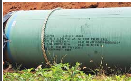
Labeling on this Mountain Valley Pipeline section shows that protective coating was applied in July 2017, 15 months before this photo was taken. Photo: NRDC
