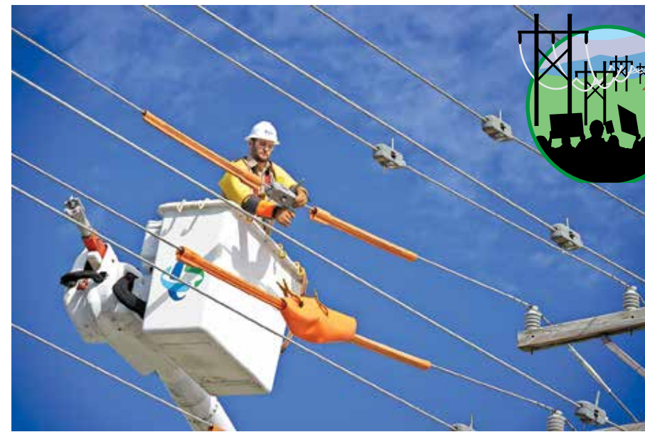
A Duke Energy lineman. Parts of Duke and Dominion Energy's grid modernization plans, which earn the utilities a rate-of-return, include projects such as burying power lines underground. Critics state that those projects are standard maintenance and should not be profited from. Photo courtesy of Duke Energy
