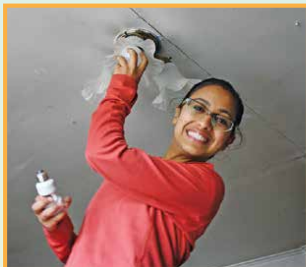
At a North Carolina home, volunteer Sadikshya Aryal replaces a CFL lightbulb with a more efficient LED one.
