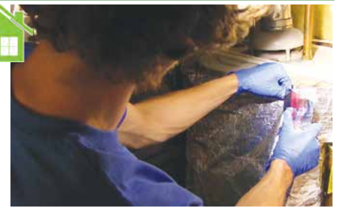
Harper Robinson of Conservation Pros connects a water heater blanket by applying insulation tape.
