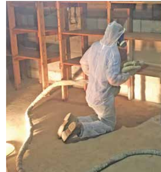
Smith Insulation contractors install spray foam in Woolery's basement. "Last year, two new [regional contracting] businesses entered the spray foam industry," says Woolery. "There's a lot of demand for this type of work." Photo by Chris Woolery.
