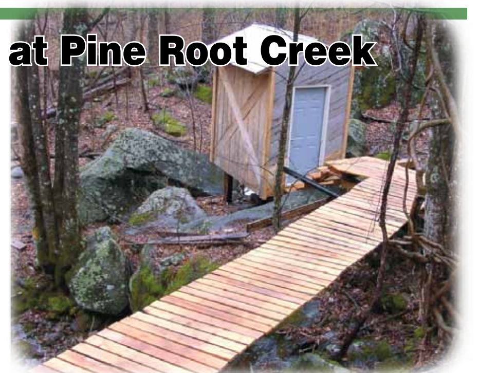
A deck leads to a shed housing a turbine and generator of Richard Cobb's microhydro system. Water is piped into the shed and the turbine creates electricity from the moving water. Water then shoots out the bottom of the shed and flows back into Pine Root Creek. Photo by Richard Cobb.
