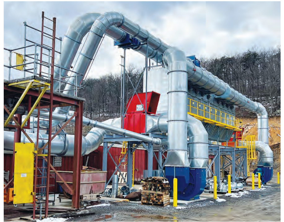
The new, highly efficient dust collection system at Gat Creek. Photo courtesy of Gat Caperton
