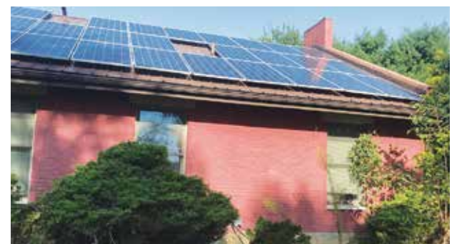
Solar panels now grace the roof of the Kuhre Center for Rural Renewal, a former coal company building in The Plains, Ohio. Photo courtesy of Rural Action
