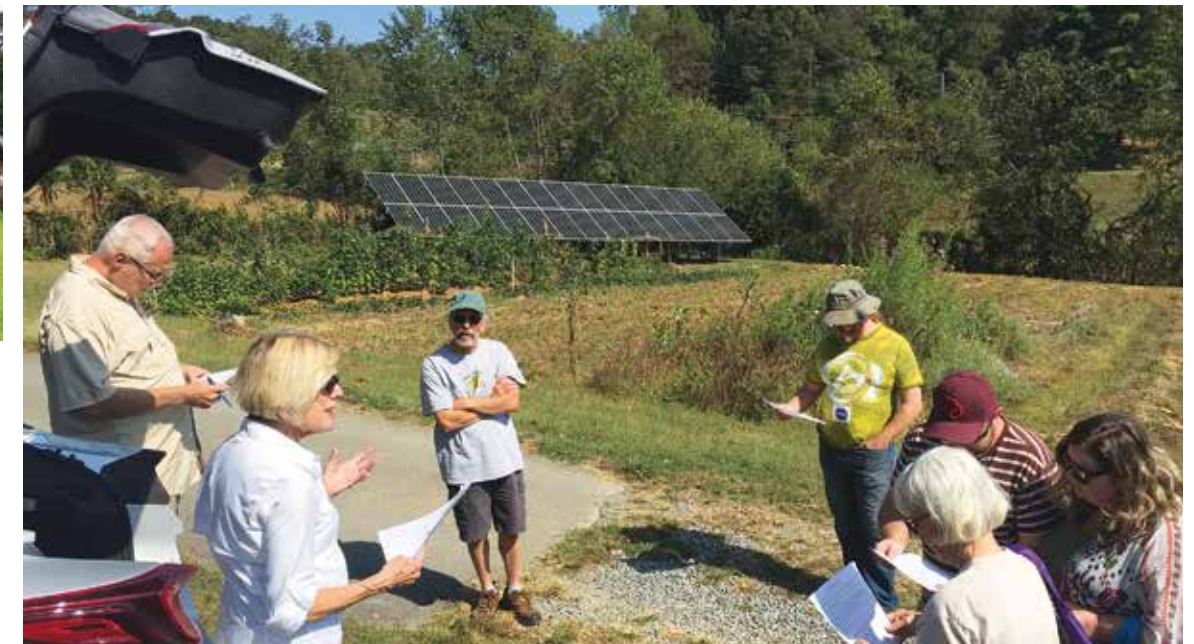
At left, Keenan Phillips stands by the ground-mounted solar panel system that powers his off-grid home. Above, Laurel Flaccavento discusses her family's solar installation with visitors during the National Solar Tour. Photos provided.
