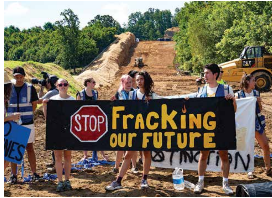
On July 20, 40 demonstrators at a Mountain Valley Pipeline construction site in Cove Hollow, Va., stalled construction for about an hour. Photo courtesy of FightingFox Photography
