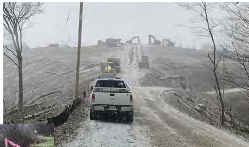
Another well pad is under construction on a ridge in Wetzel County, W.Va., above. At left, surveyor stakes mark new gas infrastructure in Doddridge County, W.Va. Photos by Dan Radmacher
