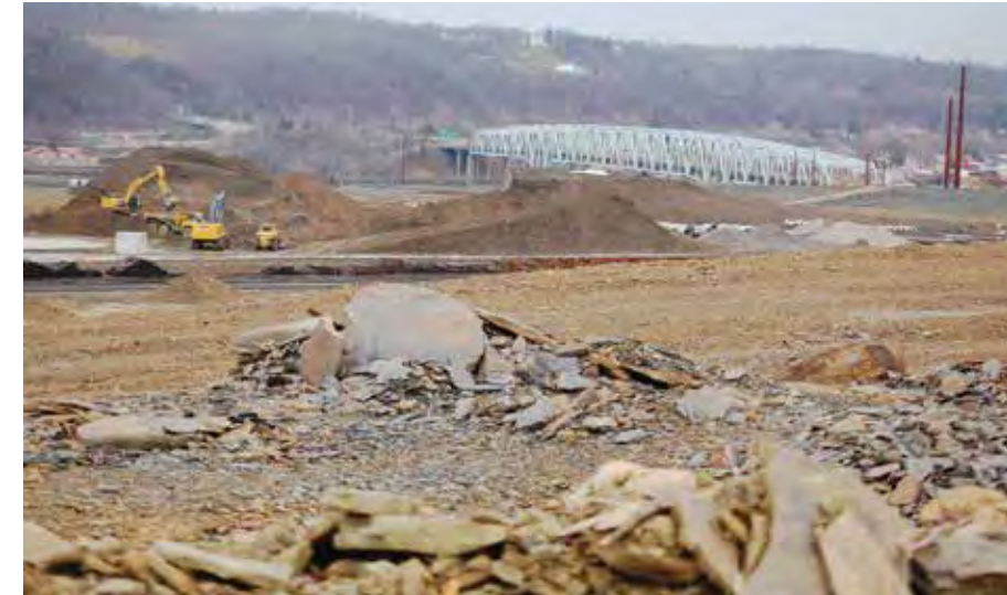
Shell began construction on an ethane cracker in Beaver County, Pa., in November. Photo courtesy of Shell Cracker Impact
