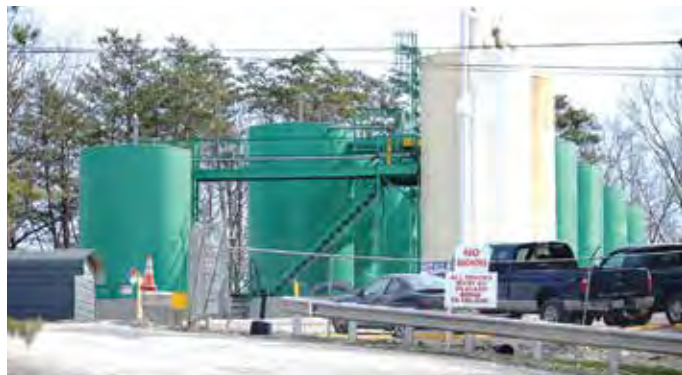
Tanks hold fracking waste at the K&H injection well site. Photo by Lorelei Goff
