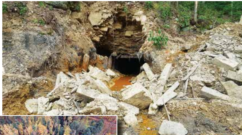
Acid mine drainage leaks from an abandoned mine, left, into West Virginia's Sovern England watershed in 2016. Photo courtesy of Friends of the Cheat. Construction on a system similar to one that treats drainage as it flows to Greens Run in West Virginia, below, will begin at the Sovern England site this spring. Photo by Adam Webster
