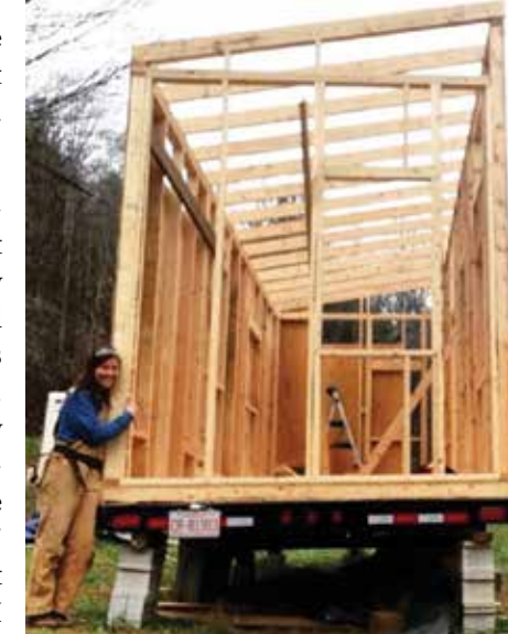
The author stands with her tiny house while working on the plywood sheathing. Photo courtesy of Sarah Kellogg
