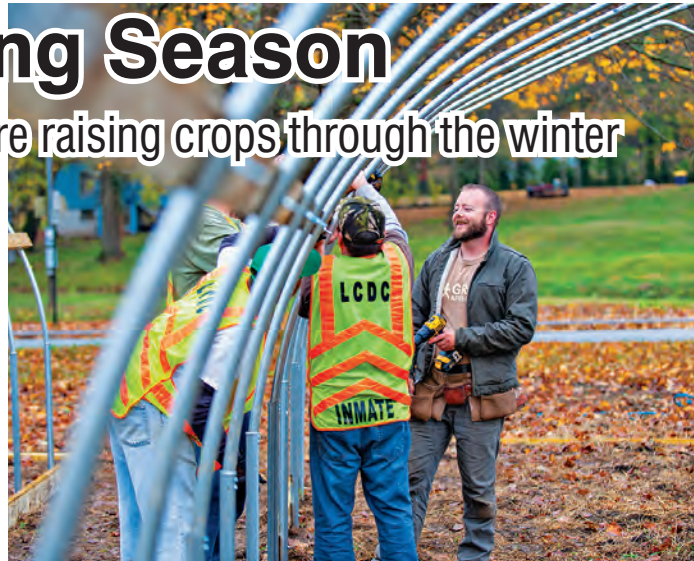
Work-release inmates help Chris McKenzie build a high tunnel for the Russellville Urban Gardening Center in Russellville, Ky. McKenzie says they were a great group to work with. Photo courtesy of the Bowling Green Daily News
