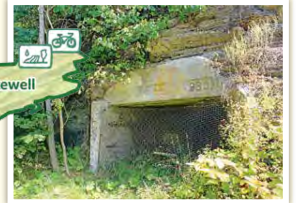
A new study shows the potential of 14 abandoned mine land sites in Southwest Virginia to contribute to the local economy. All of the sites have coal mining features, such as this abandoned underground mine portal at a proposed recreational site in Haysi. Photo by Libby Bringner
