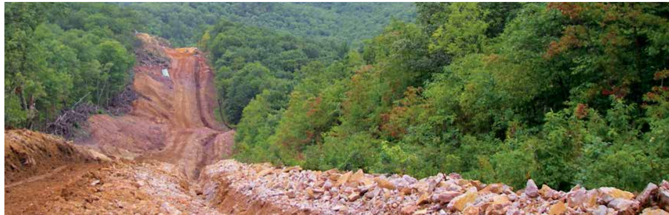
This construction corridor is wide enough to accommodate a 12-inch pipe adjacent to a 6-inch pipe. The corridor for the Atlantic Coast Pipeline and Mountain Valley Pipeline will be much wider in order to fit pipes 42-inches in diameter. Photo courtesy of Dominion Pipeline Monitoring Coalition
