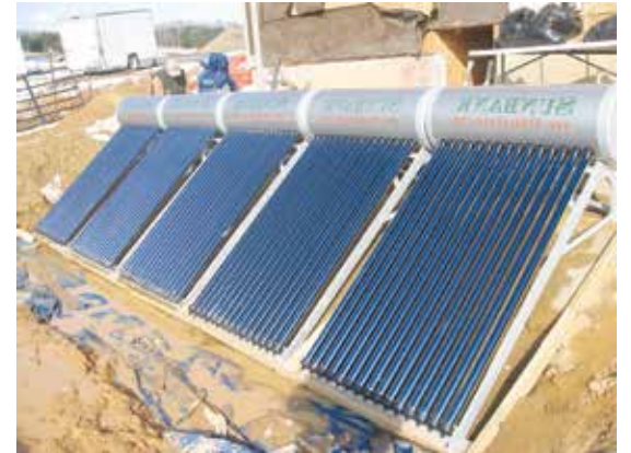
This Sunbank installation at Bethlehem Farm near Talcott, W.Va., is part of a radiant heating system on an energy-efficient house. Photo courtesy Sunbank Solar Water Heaters
