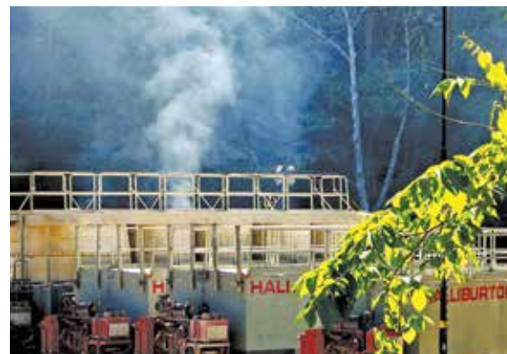
At this natural gas drilling site, one of more than 100 owned by EQT in northern West Virginia, diesel emissions from heavy drilling equipment pollute the air. Photo courtesy of Wetzel County Action Group
