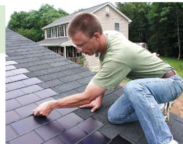
Brian Walsh installs photovoltaic panels across the state of Virginia. Photo by Pam Owen
