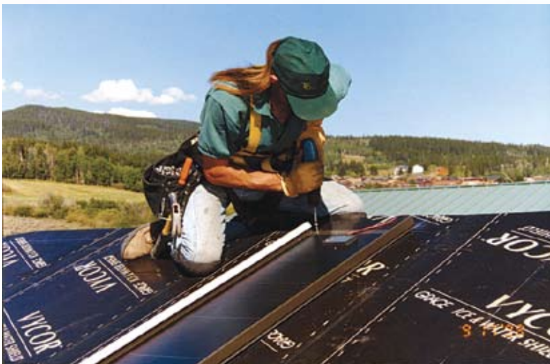
Installing a uni-solar PV roofing system. Courtesy of DOE/NREL, Credit – Joseph Burdick
