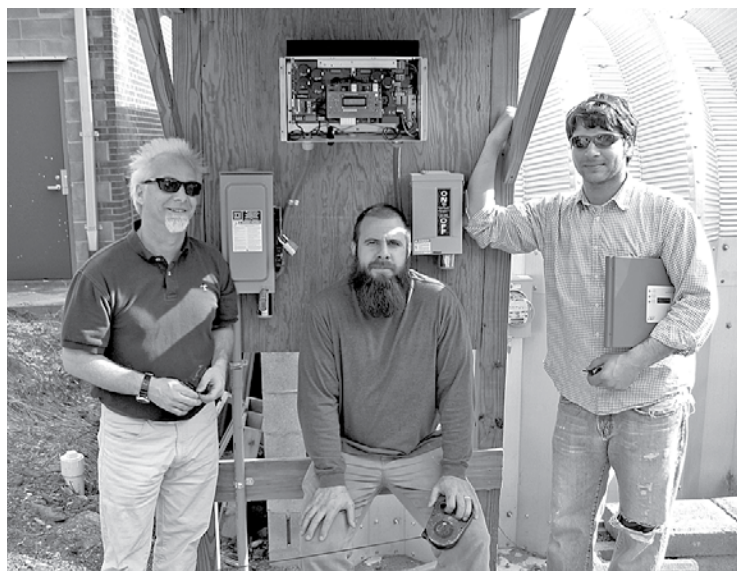
Ged Moody, Chris Crezmien and Brian Taddonio stand in front of an inverter and the grid connections for a photovoltaic system that provides power to the university's biodiesel research facility. At the time of this photo, all were students in Appalachian State University's Appropriate Technology program.
