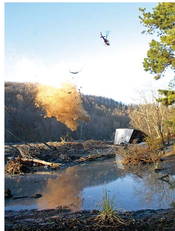
A helicopter drops a load of hay and hydroseed onto the ash near Swan Pond Circle in an attempt to prevent the ash from becoming airborne. Both ash recovery and temporary storage areas will have to be constructed before the ash can be removed from the Watts Bar Lake area. Photo by Jamie Goodman
