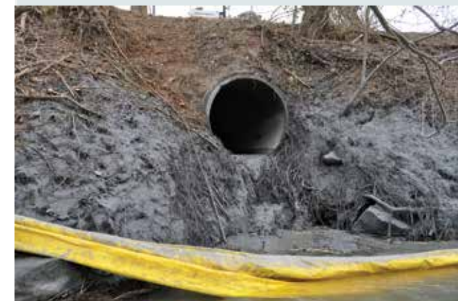
Duke Energy initially reported that the ruptured Dan River pipe was constructed from concrete. Investigations have revealed that while the visible ends of the pipe are concrete, cheaper, failure-prone metal was used for the length of the pipe. Photo courtesy Appalachian Voices
